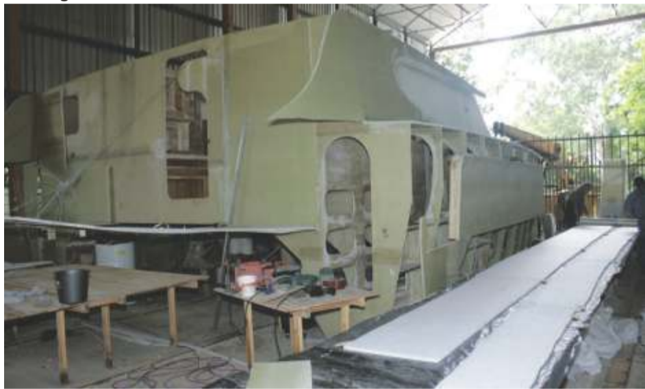
The cockpit and aft sections of the hull are yet to be installed in this pic. Behind the panel you can make out some of the bulkhead structure in the Starboard hull. Most all of the work is done from the shed floor.
